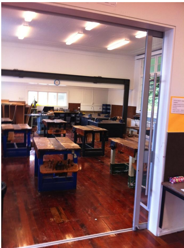
Walls removed, rooms opened with large glass sliding doors. structural beams inserted.
